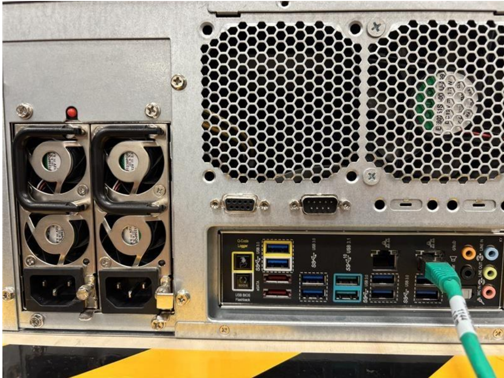
Rear system and computer I/O section
