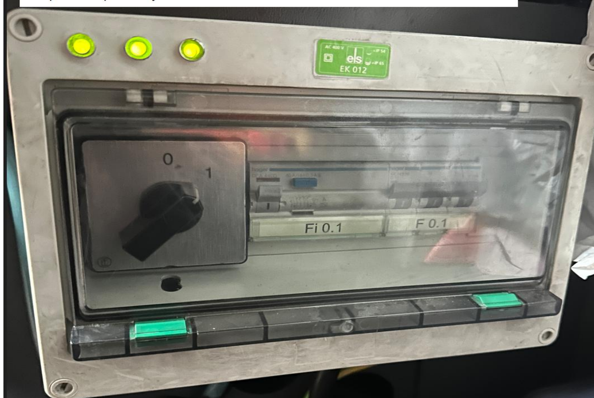
16Ampere CEE power system - main Fuses
