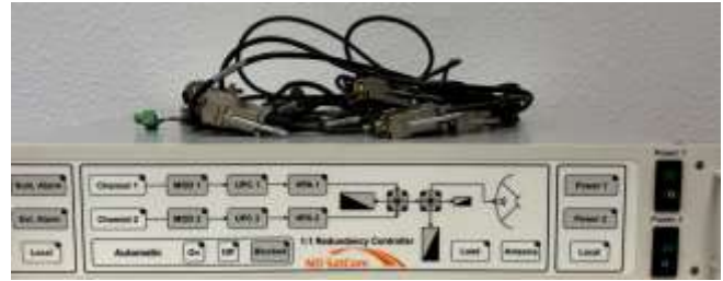
Redundancy controller with cabling
